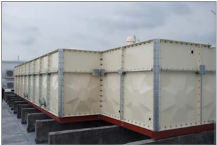
An installed FRP tank
