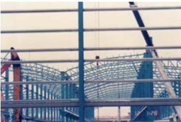
MRT C701, North Line Depot Sengkang Avenue, Singapore
